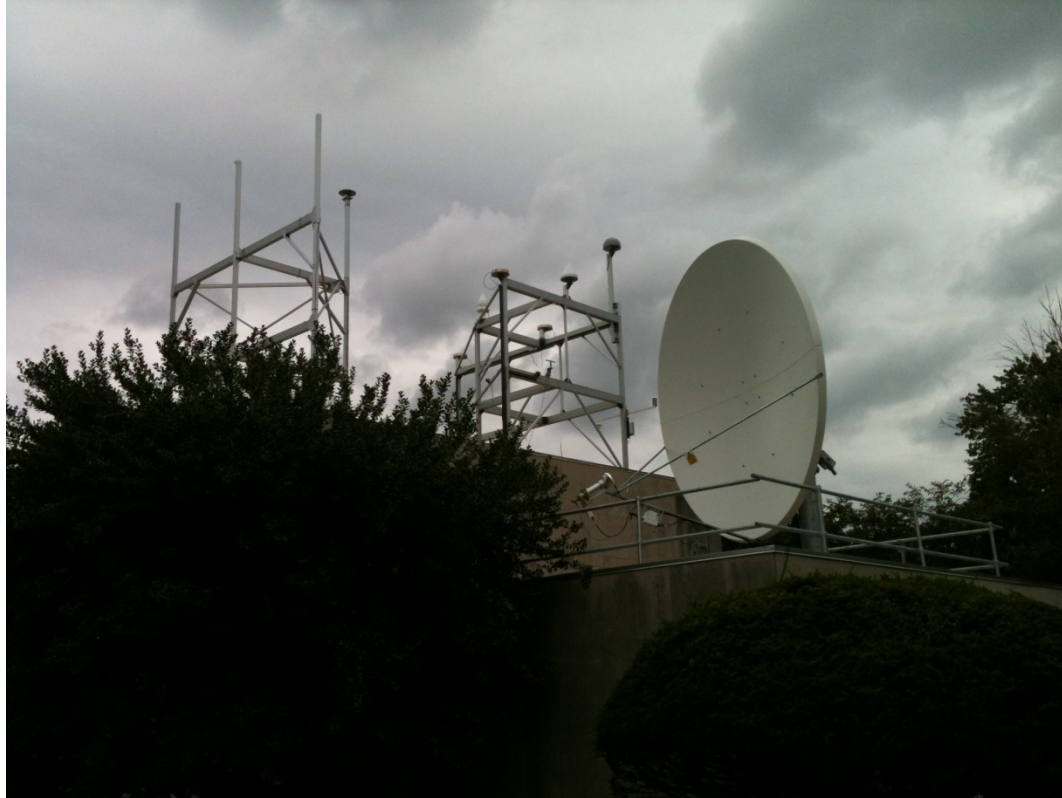
New Galileo uplink site, and masts for GNSS antennas
